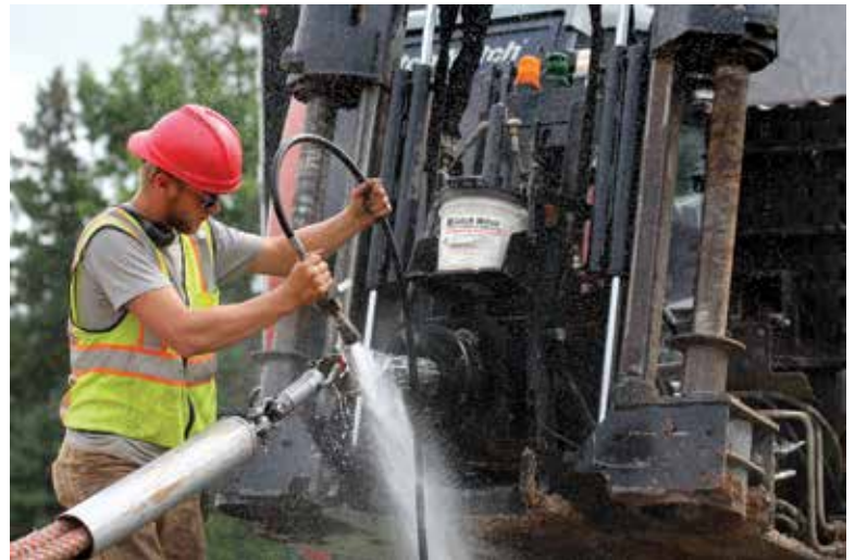
Cleaning off the directional drill components following a job will help workers keep the equipment in working condition and notice when maintenance is needed.
