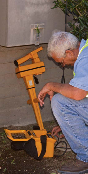
Jeff Mortenson, field supervisor, uses the Goldak Triad pipe and cable locator near the service entrance on a client's building.
