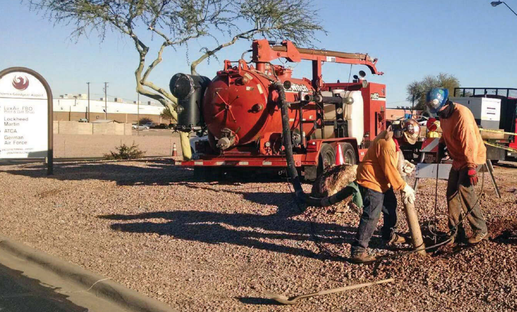
Pegasus technicians Billy Brown (left) and Jeff Williams on a vacuum excavation job with their Ditch Witch FX60, which is capable of either dry or wet excavation.
