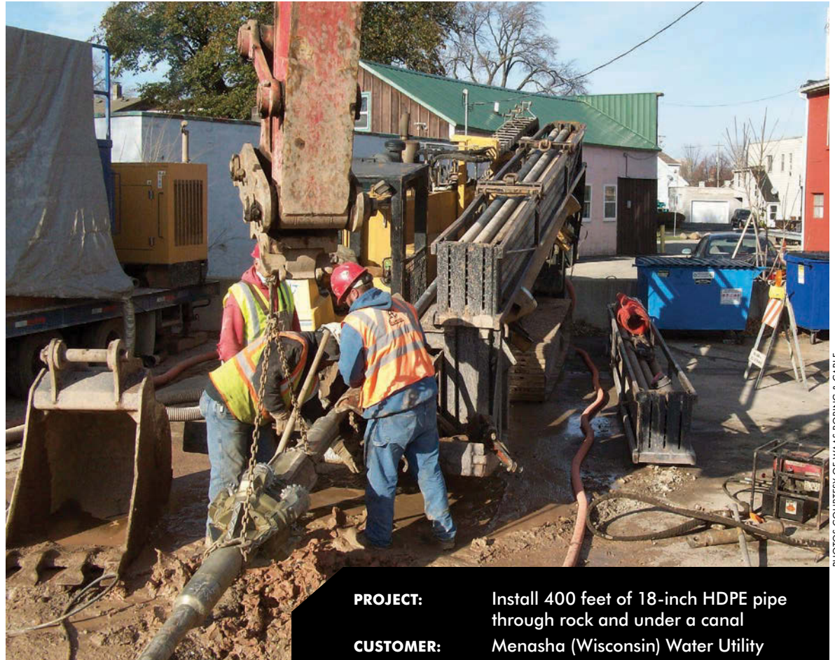
A chain and excavator boom help lift the 20-inch rock reamer as workers break apart the bore assembly in preparation for pulling drill rods to the south side.
