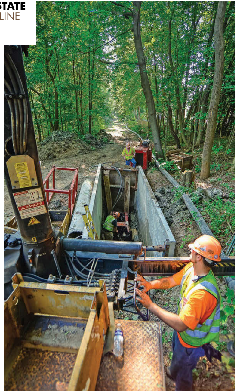
Operator Eric Gemelli operates the HammerHead HB100 static pipe bursting system to lower bursting rods into a pit. Looking on are operator Matt Bronish (in pit) and company president Matt Timberlake.
