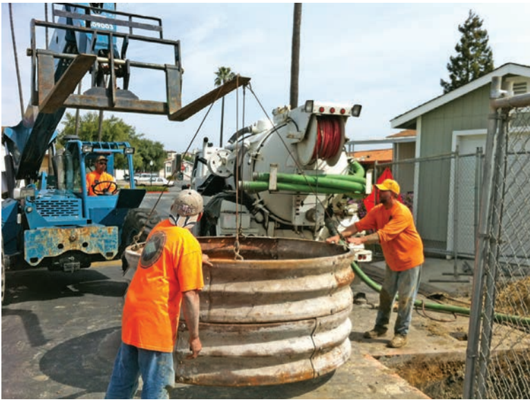
Jim Voudy (left) and John Mahana of Roddie Underground Construction help guide the 6.5-foot-diameter corrugated steel casing into place as Gustavo Barajas lifts it with the Gradall excavator.
