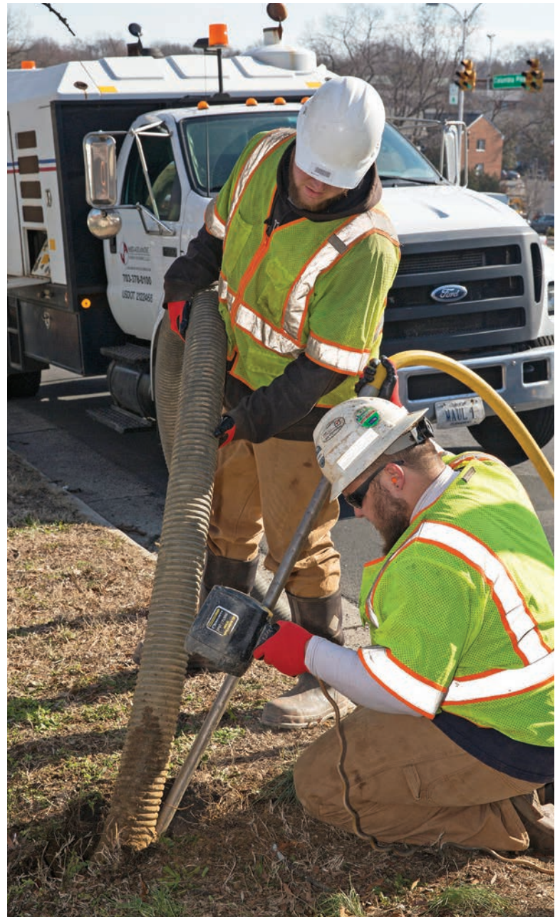
Lee Richie (left) and Stephen Russell work together to vacuum dirt and expose a utility line with the VACMASTERS 4000.
