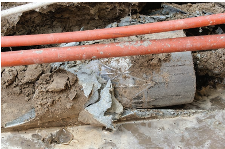
The bursting head is destroying the old pipe to make way for the new HDPE pipe.
