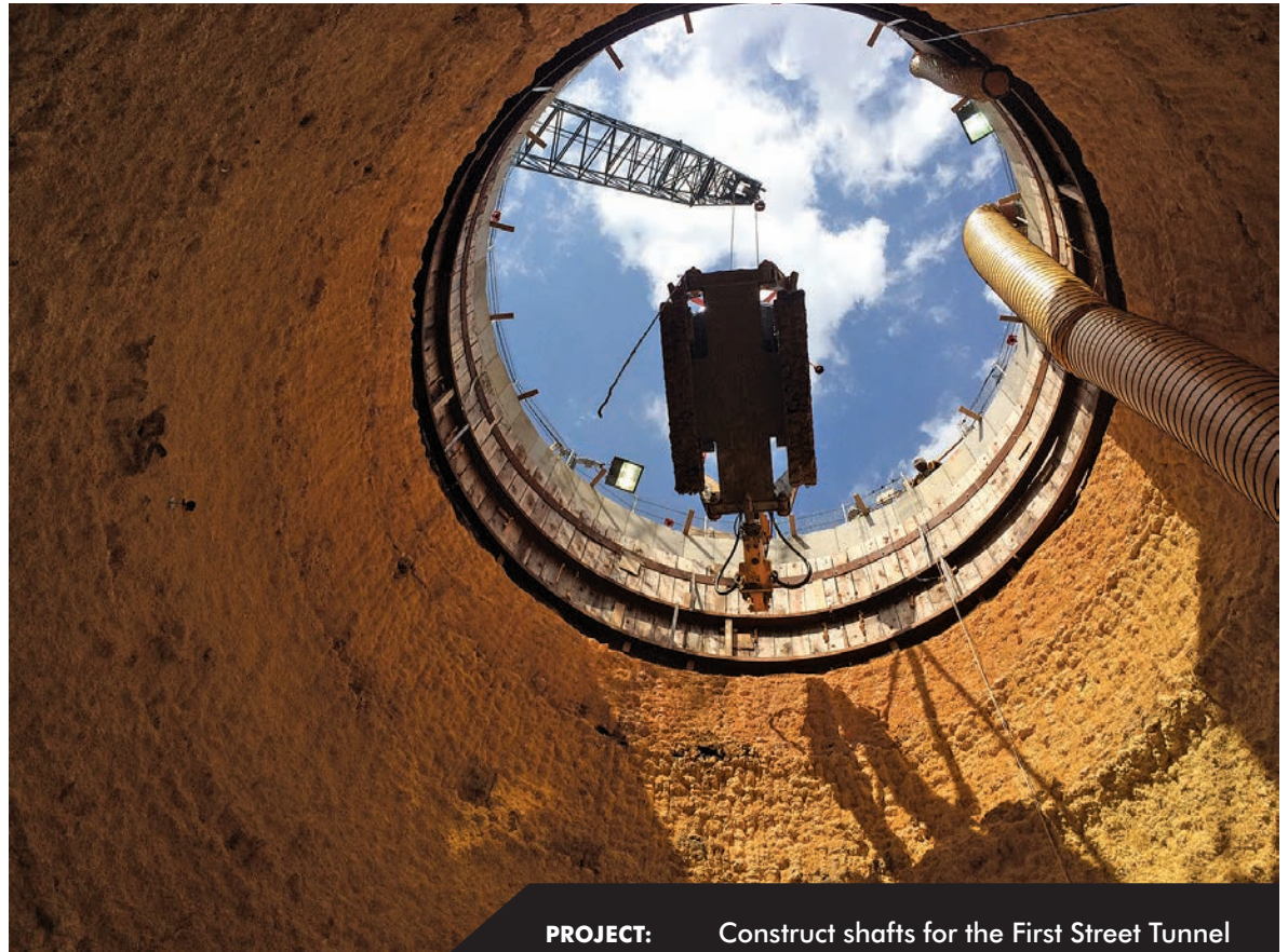
Once completed, the First Street Tunnel will stretch more than 2,700 feet, and its 21-foot-diameter tunnel can store as much as 8 million gallons of stormwater — or as much as 12 Olympic-sized swimming pools.
