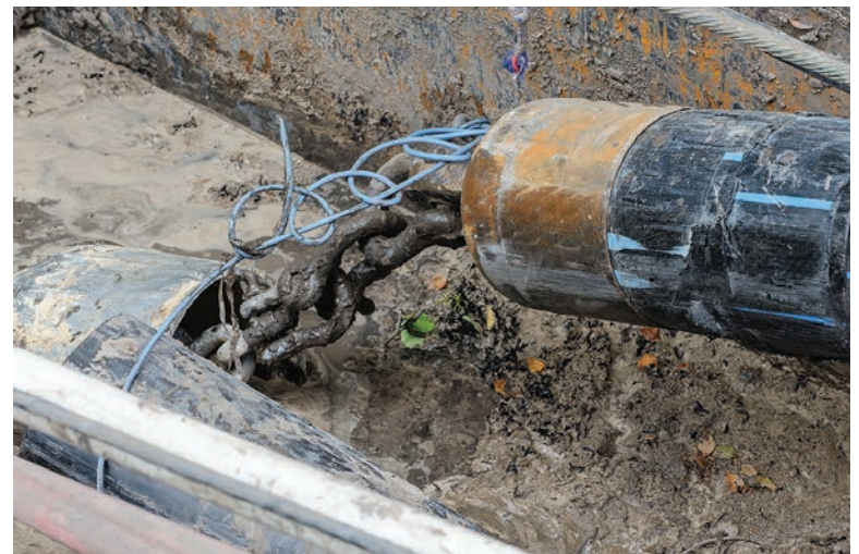
The HDPE pipe being installed is attached to the burst head and pulled into the pipe it will be replacing.
