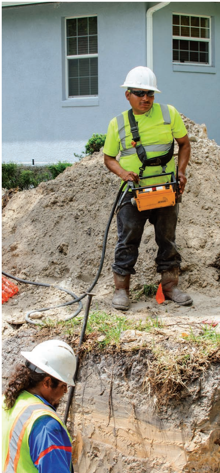
Daniel Lopez controls the TT Technologies Grundoburst bursting unit remotely with a Hetronic control, as Joshua Vasquez Morales collects the Quicklock bursting rods while on a job site in Altamonte Springs, Florida.
