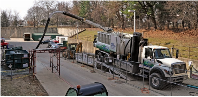
Ecotech Hydro Excavation had to park its truck across the driveway from where the work was being done and string the hose over the roadway and sidewalk to allow for vehicle and pedestrian traffic.
