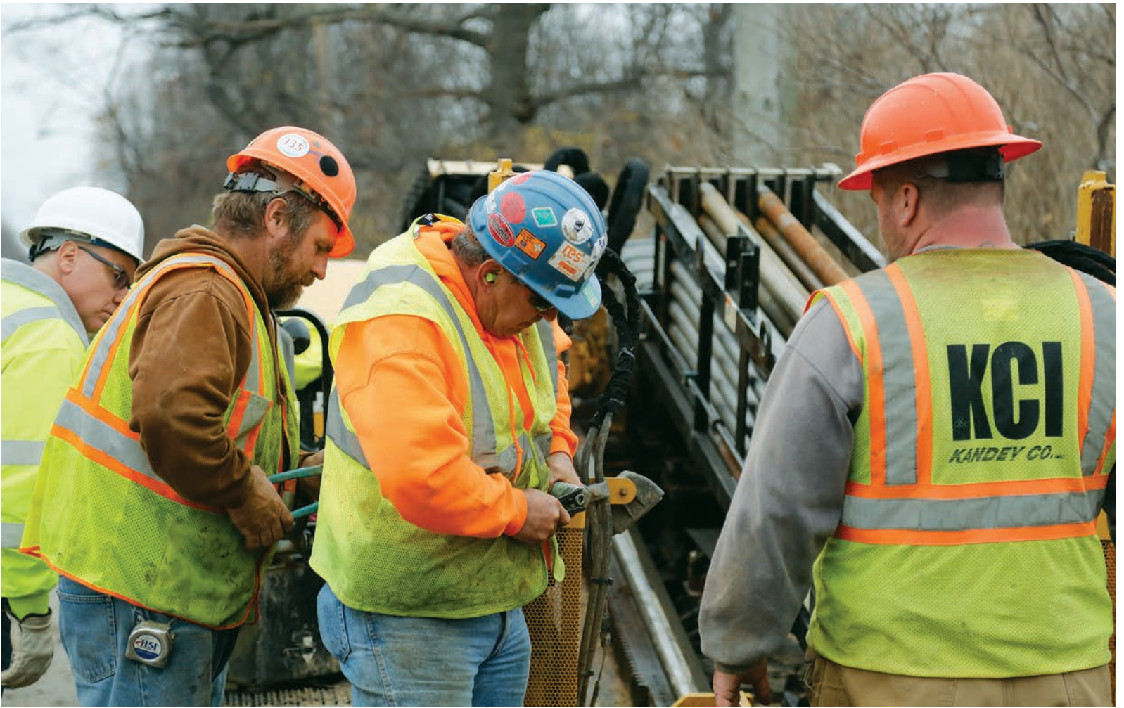
From left, James Larcara, Kandey project manager; Eric Book, labor foreman; Ron Becker, StraightLine technician; and Brad Beutner, Kandey operator, set up the directional drill on a job site.
