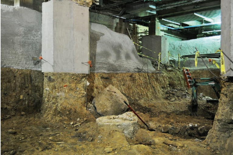
This is the work area crews from Ecotech Hydro Excavation of Pennsylvania had to contend with. Crews had to excavate under a hospital to allow it to expand.
