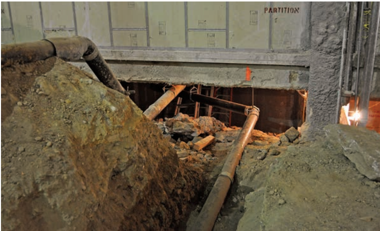
One of the challenges of the job was getting the hose into the building with a 17-foot drop at one point and a 20-foot upward incline in another. Crews also had to move the pipe through several crawlways under the hospital to get to the job site in the basement.
