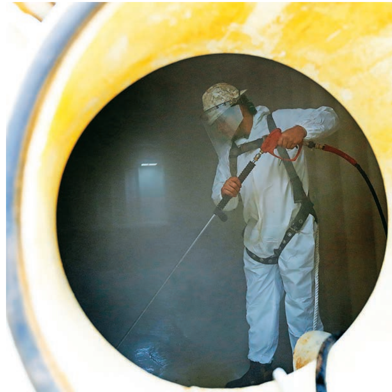
A technician cleans the inside of a steel tank with a high-pressure waterblasting unit.
