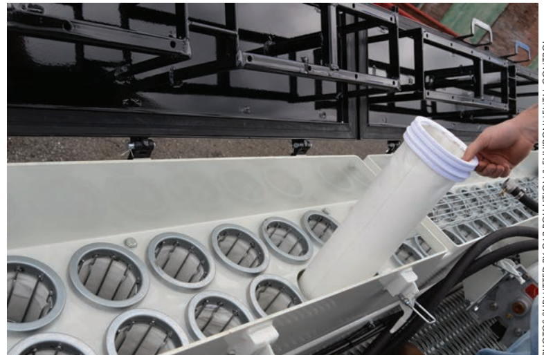
Filter bags in the baghouse are checked from the top of the hydroexcavator.
