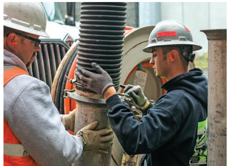
Mark Jones (left) and John Raring put the final pieces on the hydroexcavator’s boom as they prepare to excavate.
