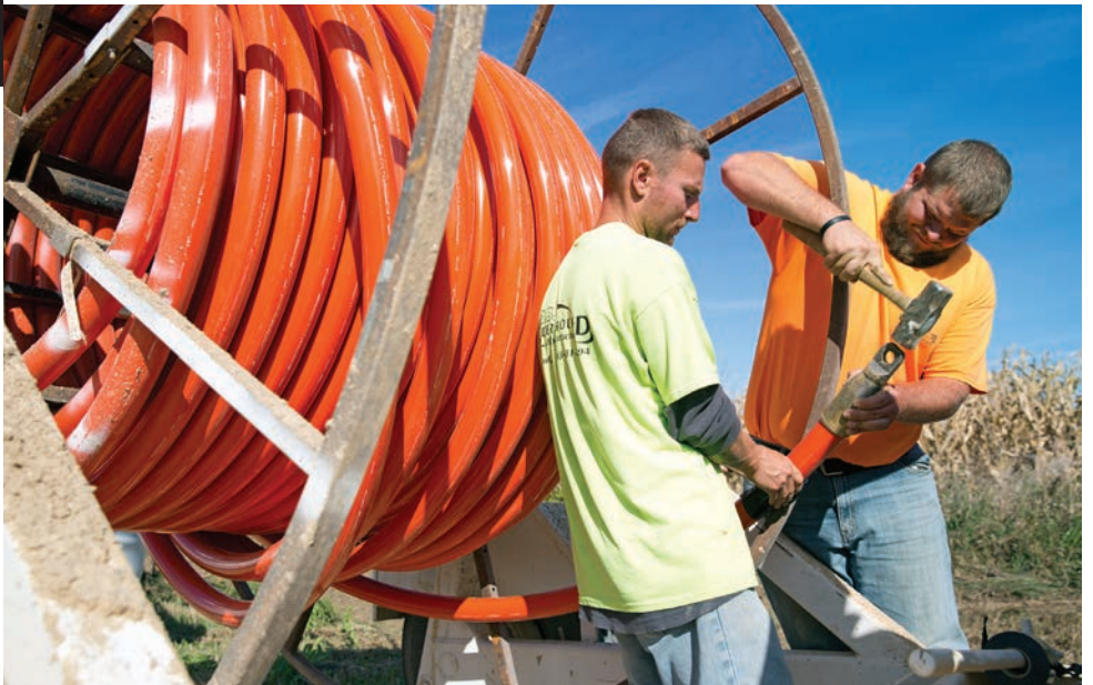
Nate Jurski (left) and Logan Heydeman prepare 2-inch HDPE conduit before attaching it to a directional drill bit.
