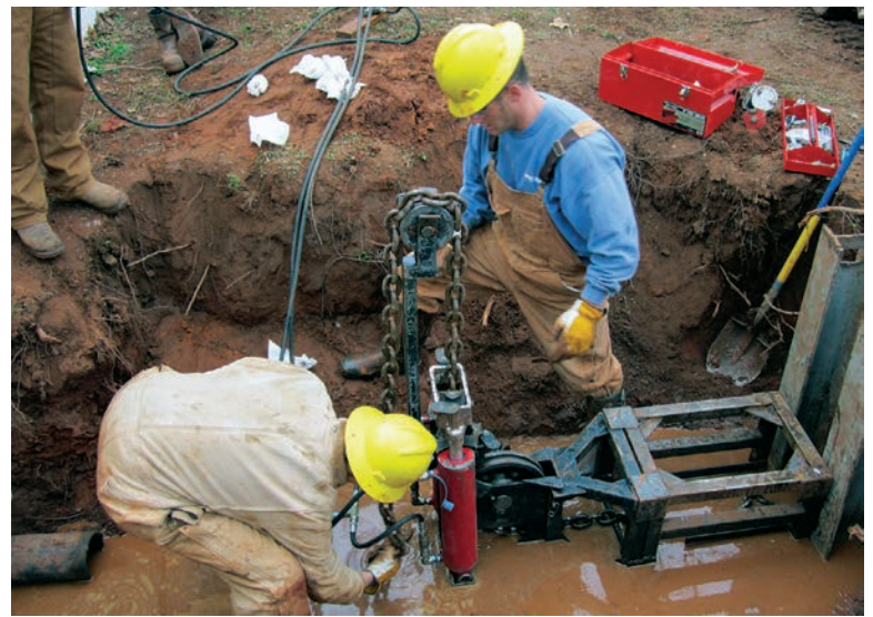
Casey Hill (left) and Jeff Cole set up the 40-ton pipe bursting system (Pipe Genie Mfg.) for the pull through the 90-degree bend under a mobile home.
