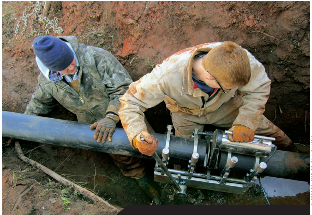
Jason Dunn (left) and Casey Hill reattach the severed 6-inch HDPE pipes with both ends in midair.
