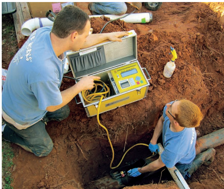
Eric Howell (left) and Casey Hill use an electrofusion processor (M.T. Deason) to install an HDPE saddle wye (Plasson).
