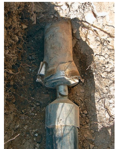
The 6-inch articulating bursting head jammed in a section of ductile iron pipe.
