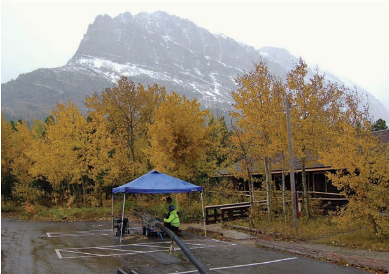
A 10- by 10-foot canopy tent keeps Pipeshark workers and the 6-inch DR11 HDPE pipe dry, as they fuse the sticks using a RODDIE portable fusion welder with a Makita-powered facing tool.
