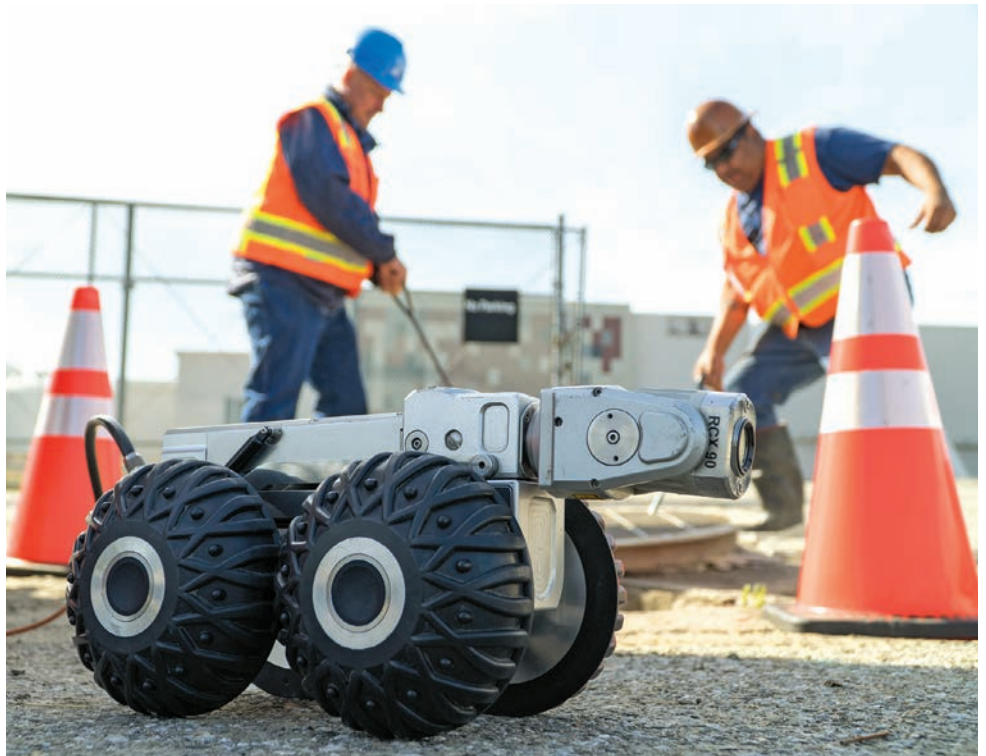
An Envirosight RX130 crawler sits on a job site in San Jose, California, where a crew from Therma Corp. prepares to use it on a sewer inspection.
