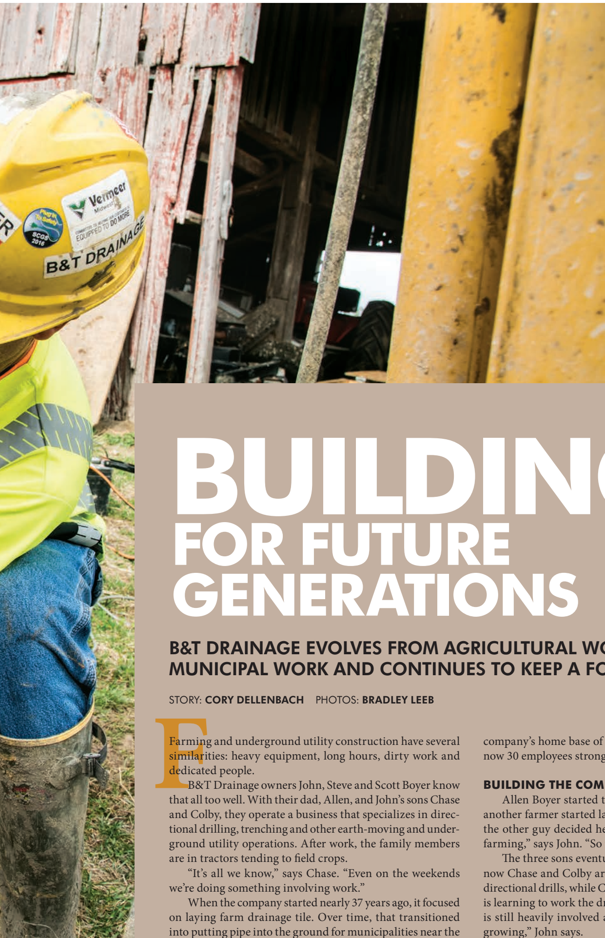
Colby Boyer, left, B&T Drainage excavator operator, and John Boyer, co-owner, work on breaking a rod free from a cutter head on a Vermeer directional drill.
