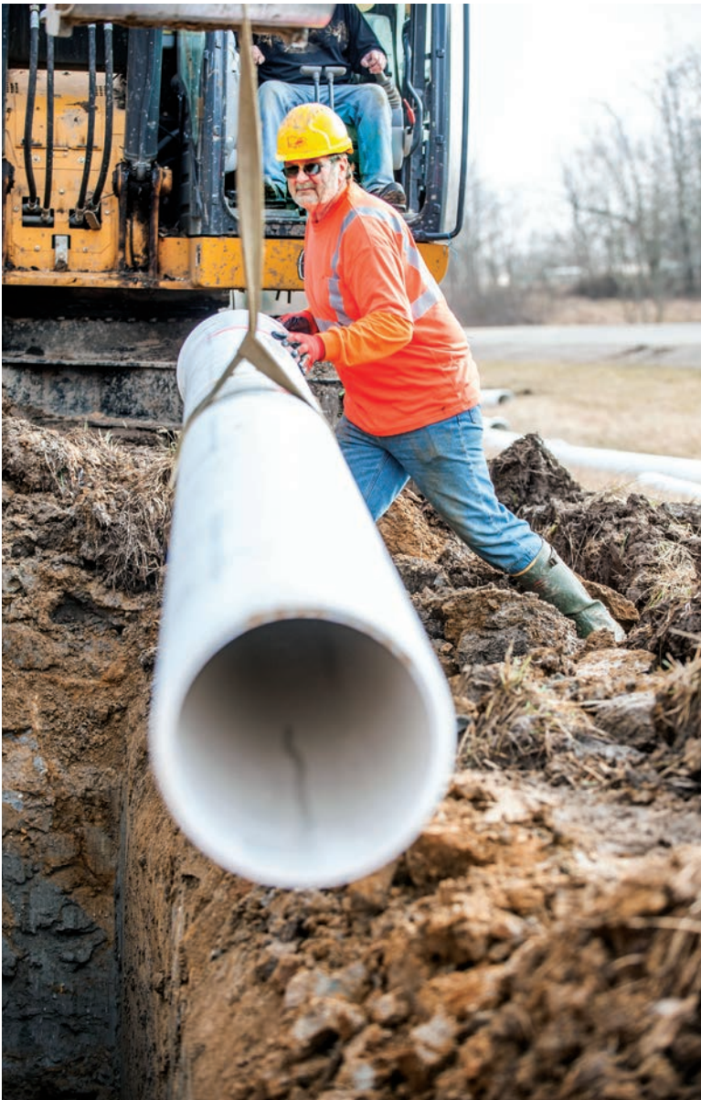
Technician Alan Lee guides a section of 12-inch PVC pipe in place.
