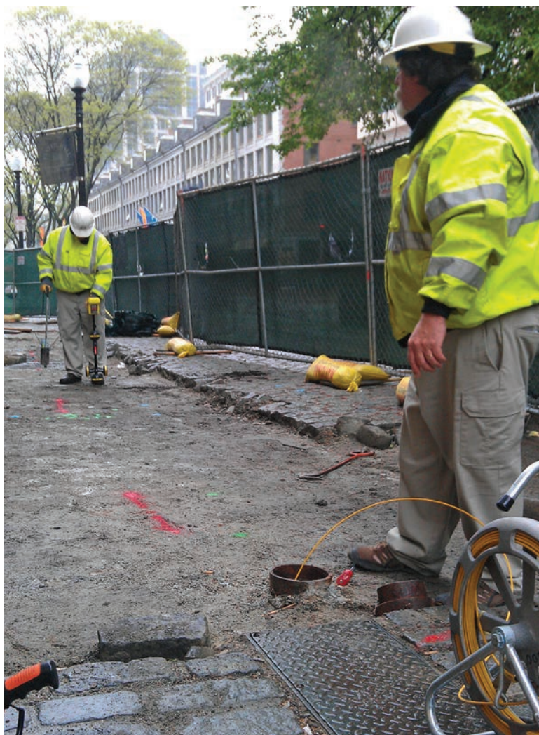
Pat Aubin, left, and Kevin Conlon locate utilities at Faneuil Hall in Boston using RIDGID locators.
