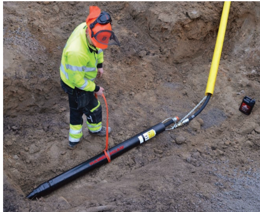
A contractor sets up a HammerHead Trenchless pneumatic piercing tool on a job. Manufacturers say the best things to remember when it comes to the tools are to clean it, lubricate it and store it correctly.
