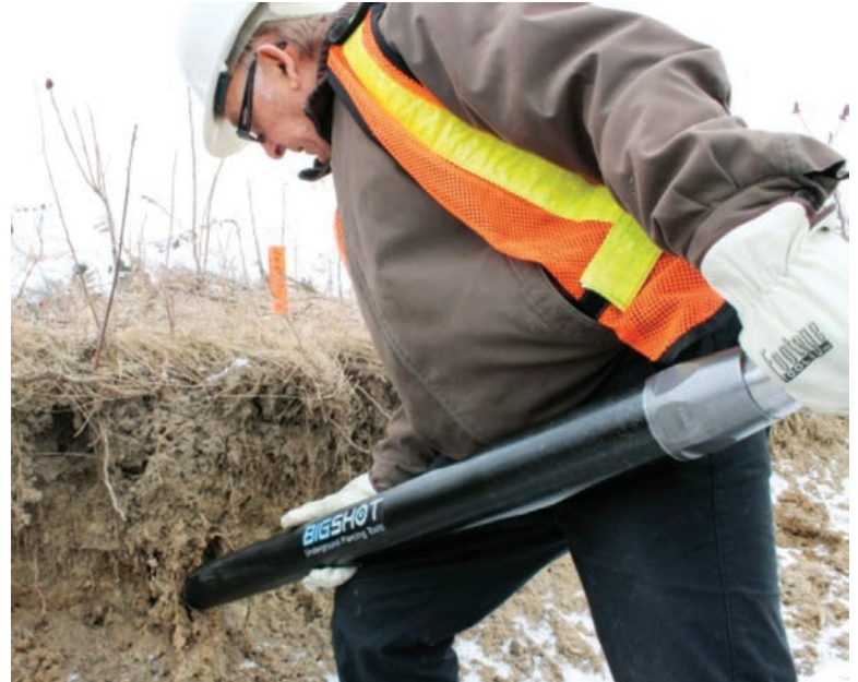
A contractor uses a Big Shot pneumatic piercing tool from Footage Tools on a job site. While piercing tools are some of the most durable pieces of equipment in the trenchless industry, contractors should still perform regular maintenance on them.
