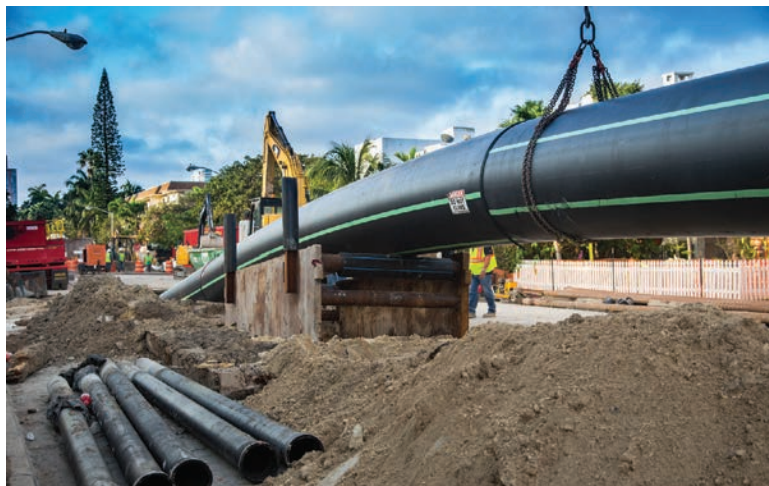
Segments of the HDPE pipe being put in at Miami Beach, Florida, rest on top of shoring devices to help it get the correct angle heading into the pullback hole.
