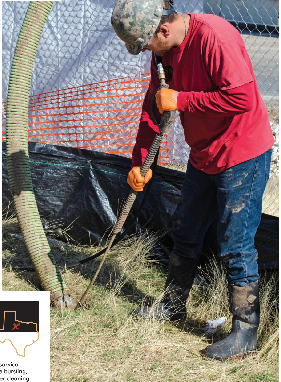
Jason Sherman uses the wand of the Ditch Witch FX30 hydrovac trailer unit to break up the ground during a job in Abilene, Texas.
