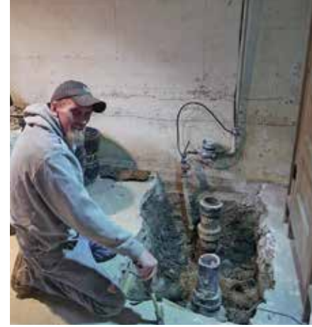
A technician from Skooters Plumbing and Drain Cleaning in Fargo, North Dakota, prepares for the new waterline and sewer line to enter the house. Crews installed a new 1-inch copper waterline and a 4-inch HDPE sewer line.
