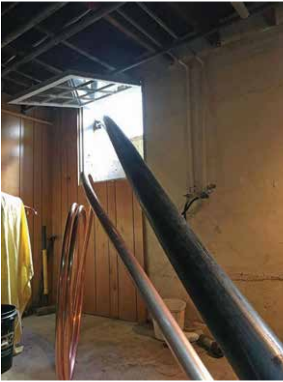
Both the copper waterline and the HDPE sewer line enter the basement of the home as they are pulled back through the old pipe.
