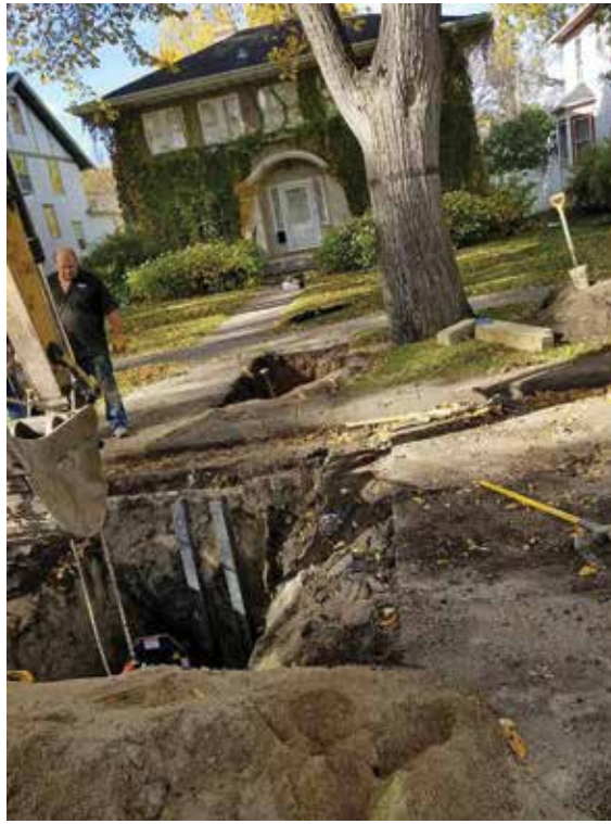
The entry pit for the pipe bursting job in Fargo, North Dakota. Skooters Plumbing and Drain Cleaning handled everything from the excavation to the pipe bursting, including patching up the road and basement.
