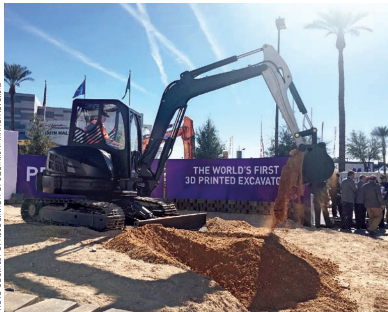
The 3D excavator on display and in action at CONEXPO-CON/AGG and IFPE 2017 in Las Vegas.
