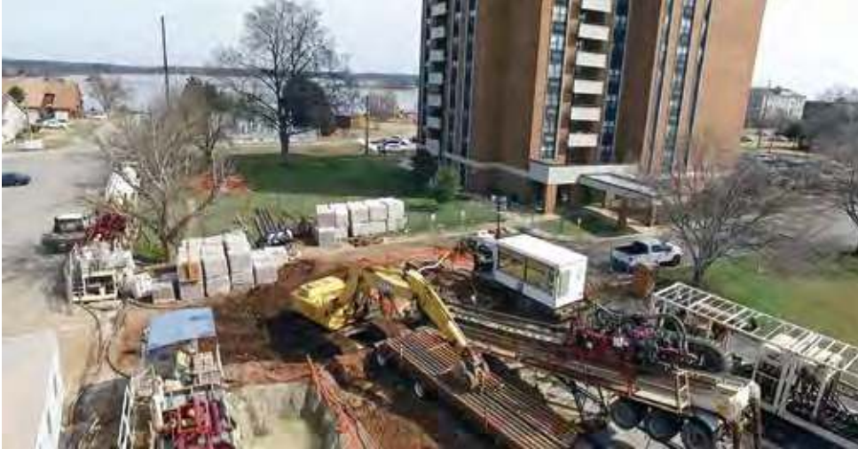
A 1.1-million-pound American Augers directional drill sits at the entry pit of the 3,000-foot-long HDD project involving digging under Wheeler Lake in Alabama. The entry pit was in the parking lot of a retirement home.
