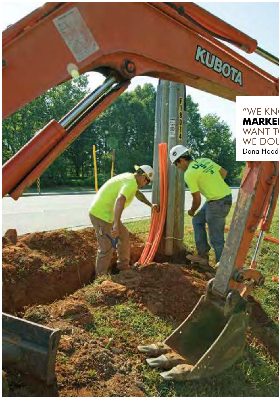
Jeremy McGee (left) and Everett Skeen install conduits for a major telecommunications company to upgrade their fiber optic backbone in an area that is currently being served by old copper cables.
