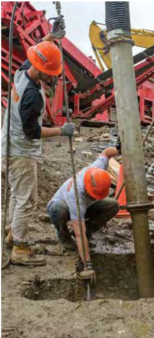
J. Angelo Industries takes pride in handling every facet of an underground problem.
