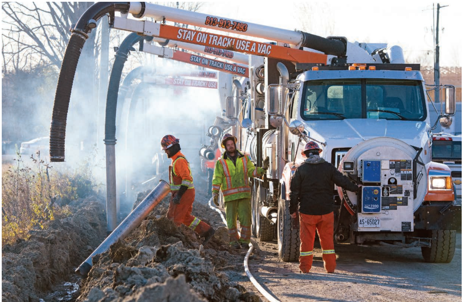
NCM Hydro Vac Services operators dig with the fleet of Vactor 2100s outside the company shop in Ottawa, Ontario.
