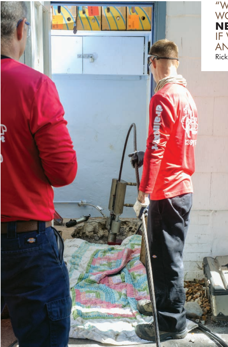
Rick Hedge (left) operates the TRIC Tools bursting unit as Jason Pegg guides the cable exiting the pit.
