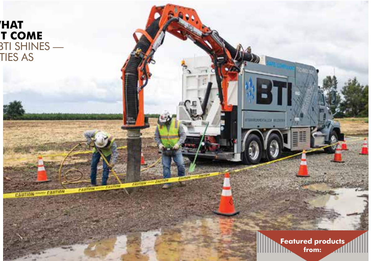
BTI boasts seven dry-suction Dino excavator trucks (MTS GmbH; distributed by OX Equipment) and 75 employees. The company offers dry-suction excavation services, transportation and disposal of hazardous and nonhazardous waste, and frac-tank rentals.
