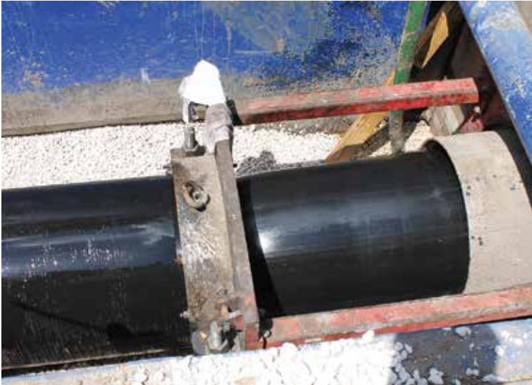
The method of compression pipe-lining with HDPE pipe technology was brought to the U.S. from England in 1999.
