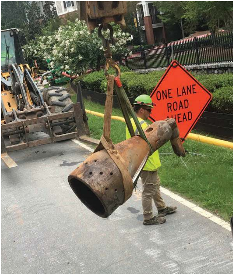
The pipe bursting project at Kennesaw State University required a significant upsized from 10-inch vitrified clay pipe to 16-inch HDPE. Shown here is the pipe bursting expander.
