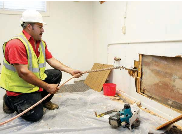
Technician Martin Salazar prepares the copper waterline in the house for a pullback with the directional drill outside.
