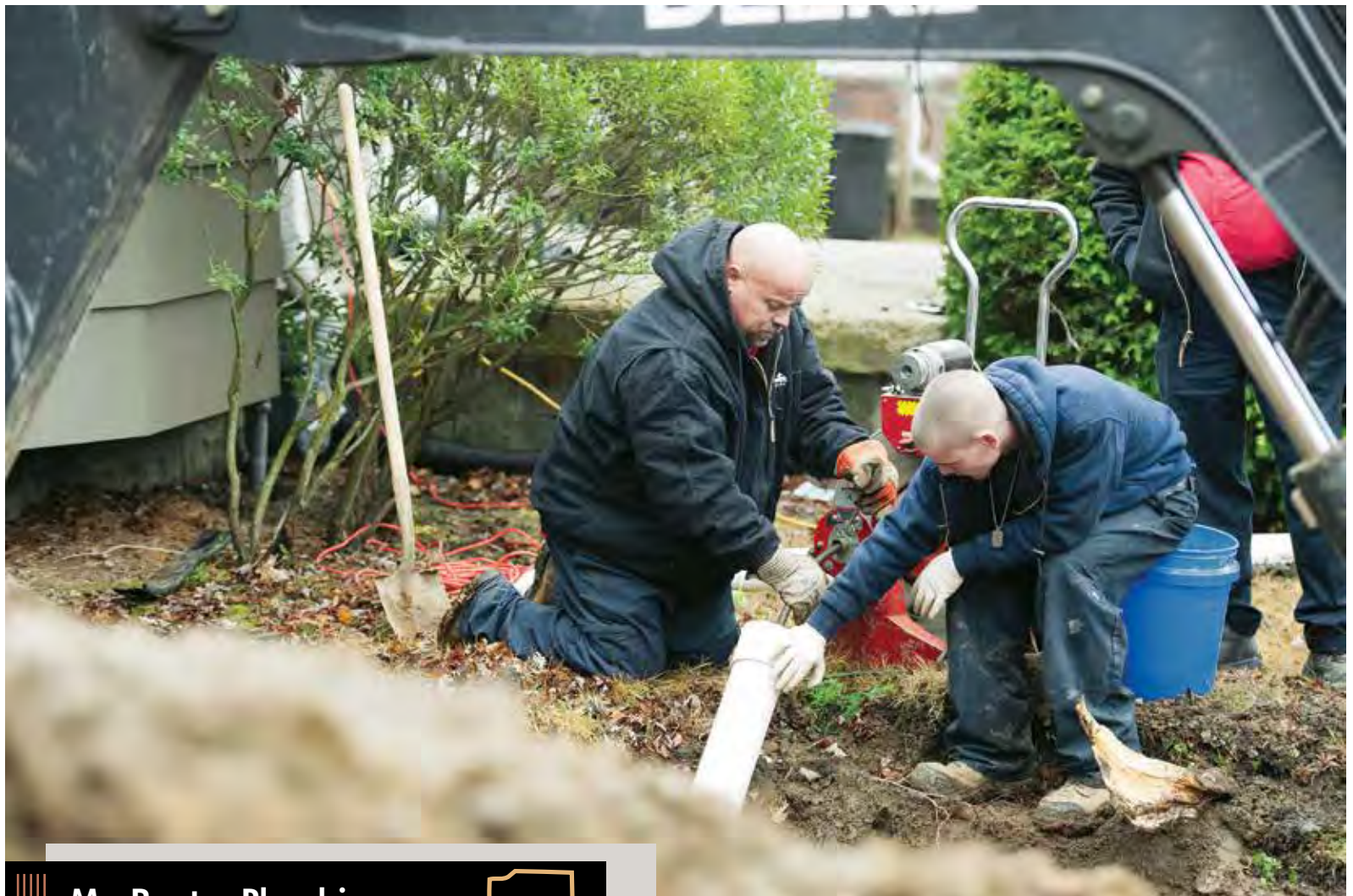
Jonathan Wilhelm, right, apprentice, and Robert Wilhelm, field manager, use a Spartan 1065 cable machine to remove roots from a residential sewer line in Indianapolis.
