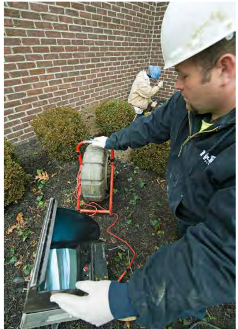
Carrig watches the monitor of the Spartan SparVision 200 sewer video camera as Glen Ethridge, excavation tech, feeds it down into a residential sewer system.
