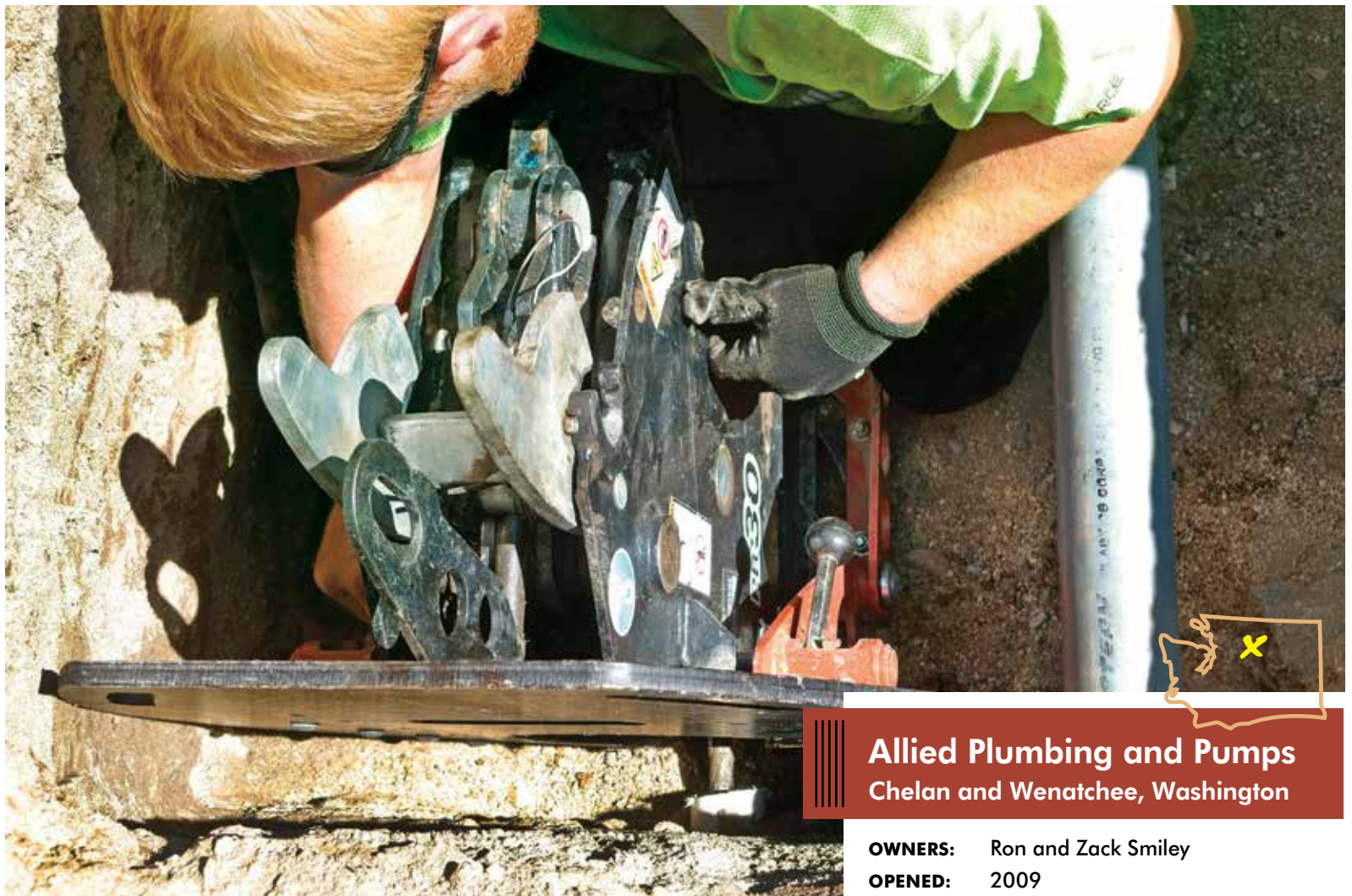
Korey Kase of Allied Plumbing and Pumps installs a pipe bursting machine (HammerHead Trenchless) in preparation for a new sewer line to be pulled through the existing line.
