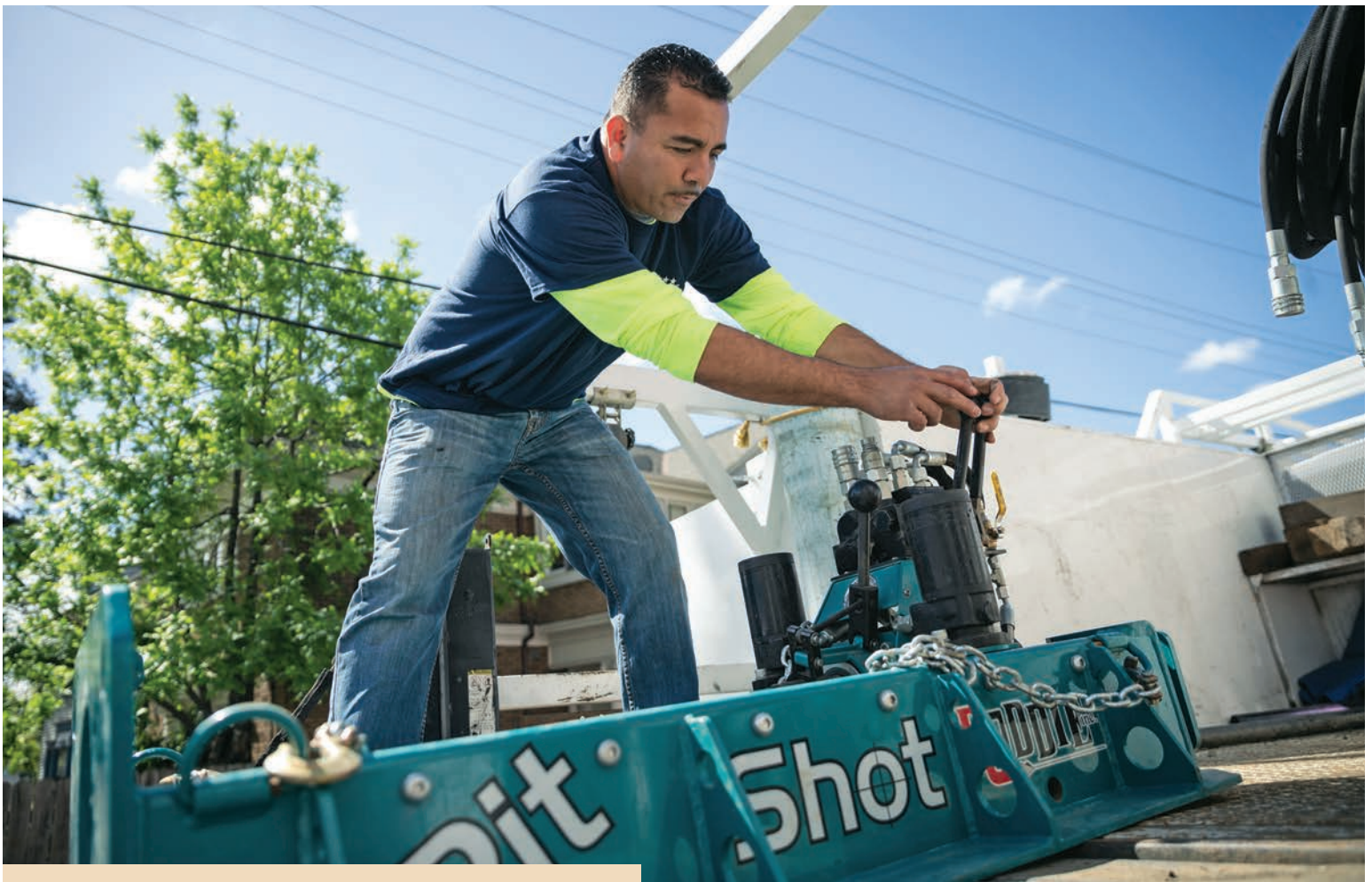
Ray Ramirez, one of the first in the area to invest in pipe bursting and repair equipment, sets up a RODDIE Pit Shot directional drill on a job site.
