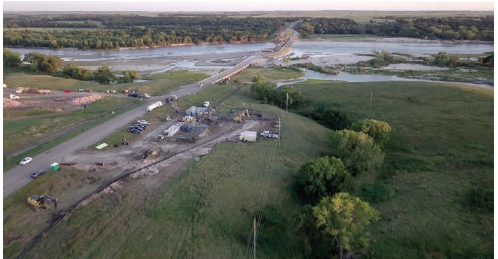
An aerial view of the job site from one side of the Niobrara River looking across to the other side. Crews had to drill a 4,320-foot bore under the river to replace a failed waterline.
