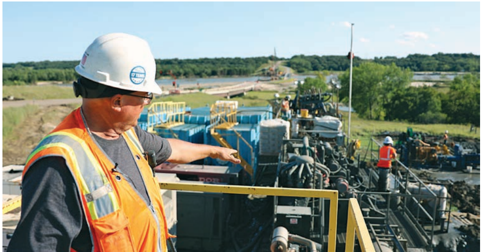
A contractor from Horizontal Boring & Tunneling gives an overview of the job site at the entry pit.
