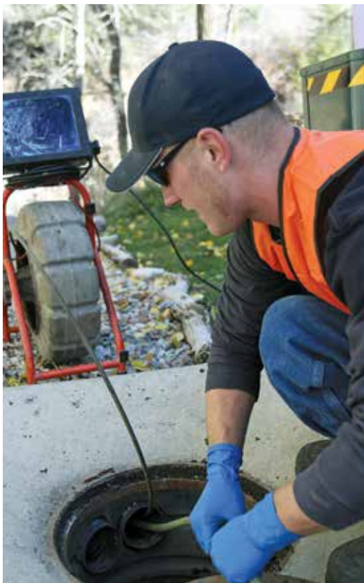
Adam Crambell feeds a video camera (RIDGID) through a pipe as he watches the video monitor to check for blockages in the lines during a jetting service call.
