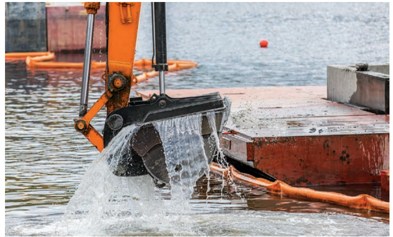
The buckets of the excavator have an environmental lid, which is a 60-inch-wide steel plate that hydraulically closes over the bucket and secures the sediment within it.
