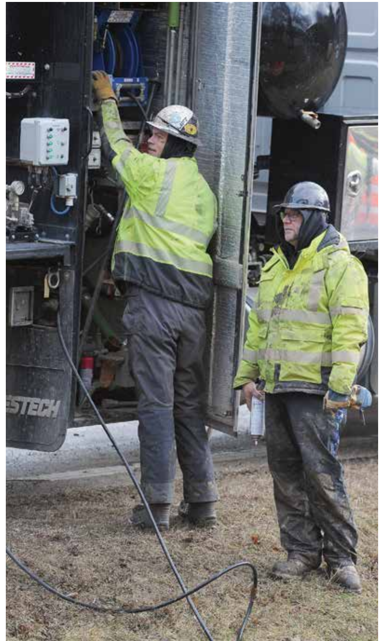
Ben Horaitis, left, hydrovac operator, and Bill Lietzke, company owner, get the hydroexcavator ready for a job near Milwaukee. Lietzke still enjoys getting out and working with his crews as often as possible.
