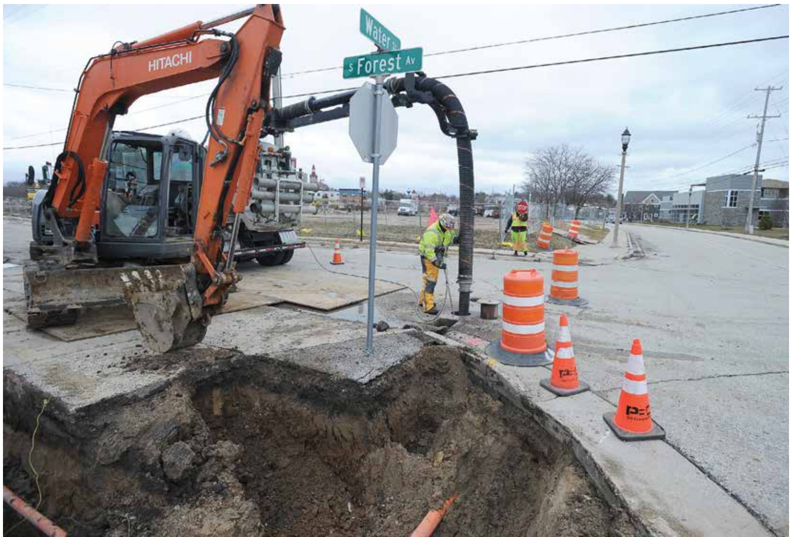
Louie Kelly potholes for utility lines at a Milwaukee intersection, where street work is occurring. The company marks off an area where they are working and has a crew member directing traffic for further safety.
