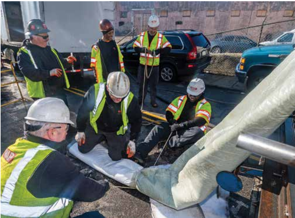
The team from North American Pipeline prepares the pipe liner to be used on a repair job (Applied Felts). Pipe lining and replacement is a growing side of the company's business.
