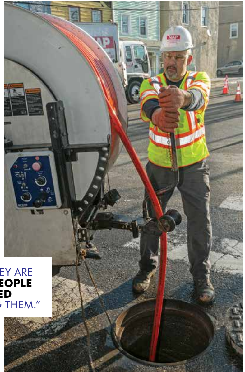
Jerzy Pleskowicz uses the Vector 2100 sewer cleaning truck to lower the jetter into the sewer drain.
