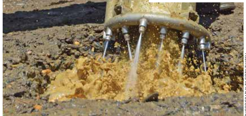
North American Pipeline Services operator Ray Regan uses a Vactor 2100 Plus hydroexcavator on a job site near Freehold, New Jersey, using a dig tube from Soil Surgeon.
