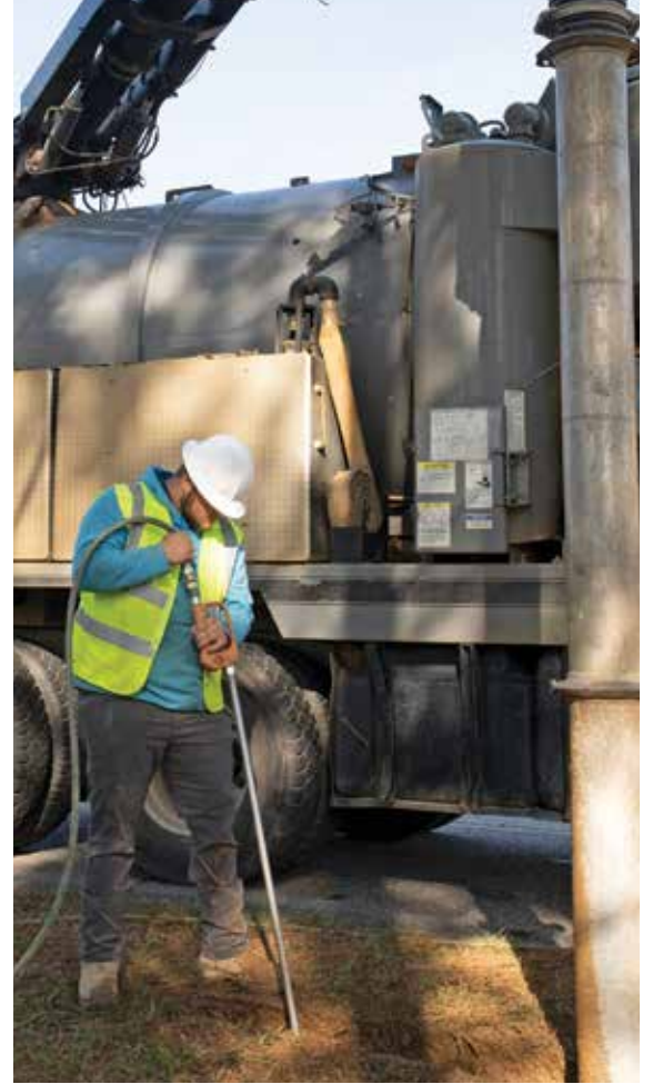
Hydroexcavator operator Tristan Hood uses a digging wand from the Vac-Con truck to expose utilities ahead of the directional drill being used.
