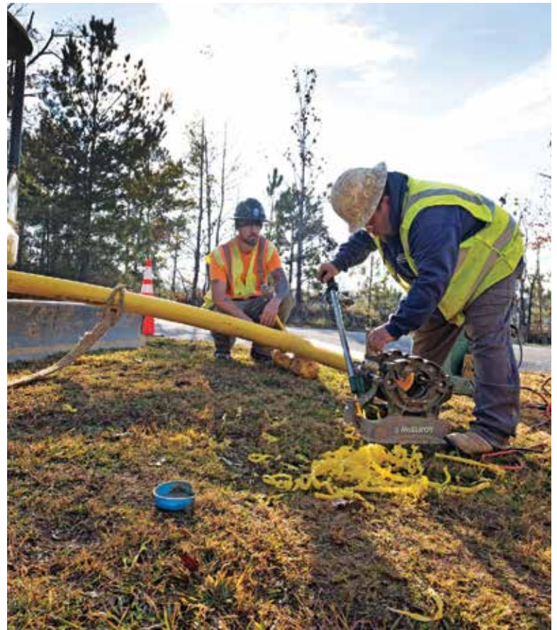
Philip James (left) and Josh Burr use a McElroy 4-inch butt-fusion clamp as they connect gas pipeline. They use a shaver to make the end flush to allow for a proper and quality fuse.
