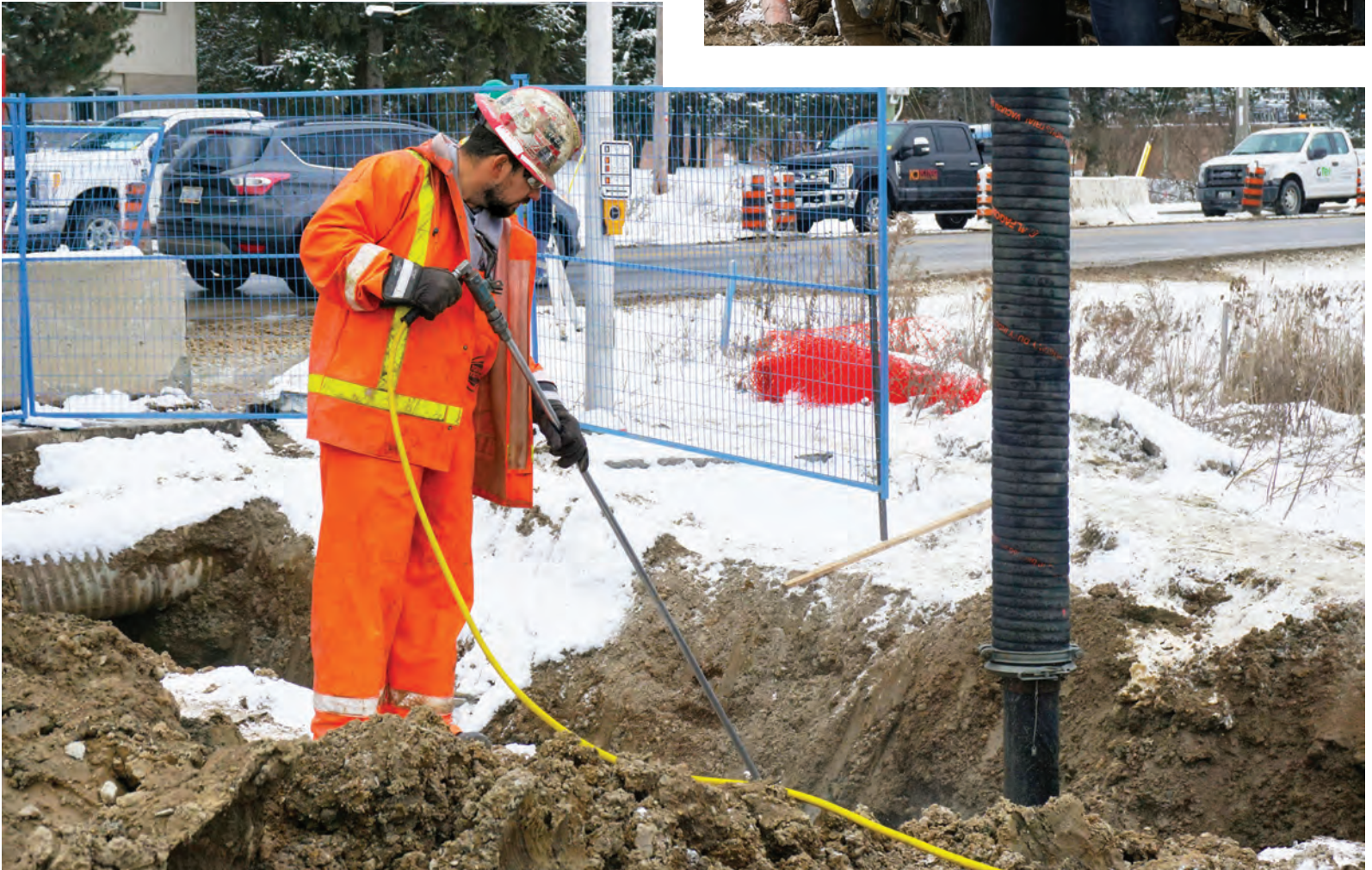
Hydrovac driver Luis Farias uses the digging wand from one of the company’s three Tornado hydroexcavators to expose utilities prior to a directional drilling job.
