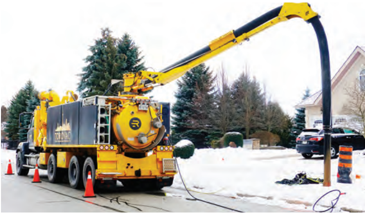
Torovac Services boasts four Rival T10 hydroexcavators with plans to add another to the fleet later this year.
