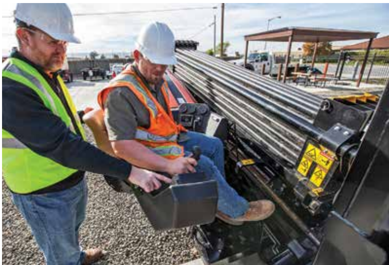
A contractor is getting some instruction from a Ditch Witch trainer while on a directional drill. One way that manufacturers like Ditch Witch are supporting the workforce is through maintaining machine design and consistency across contractors' HDD fleets.
