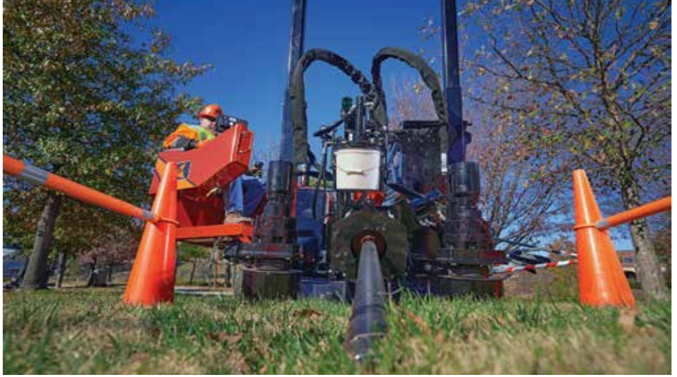
A contractor uses a Ditch Witch drill on a job site. Aside from controls and electronic interfaces, some manufacturers offer the same drill operation across their pipe and tooling, features, operator platform and overall machine design.
