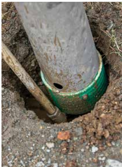
Educating customers on the benefits of vacuum excavation work is important to HydroEx as the only vacuum excavation company on the island.
