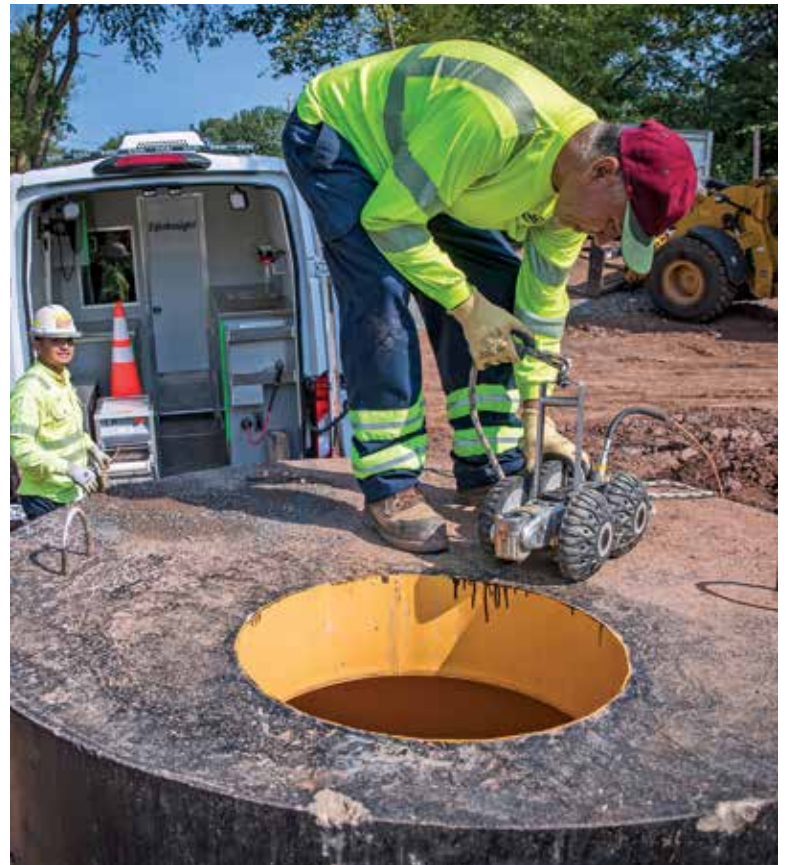
Quality Pipe Cleaning doesn’t only do excavation work, the company also offers services such as pipe cleaning and CCTV. Here technicians Erik Rodriguez (left) and Patricio Carillo prepare to lower a Rovver X 130 (Envirosight) into a manhole for inspection for a storm retention system.
