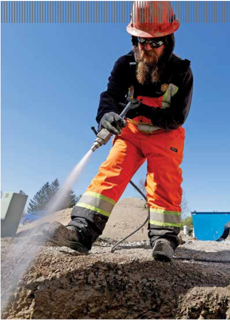
Carmon Geffs uses the digging wand from the hydroexcavator to loosen the soil for the trenching operation.
