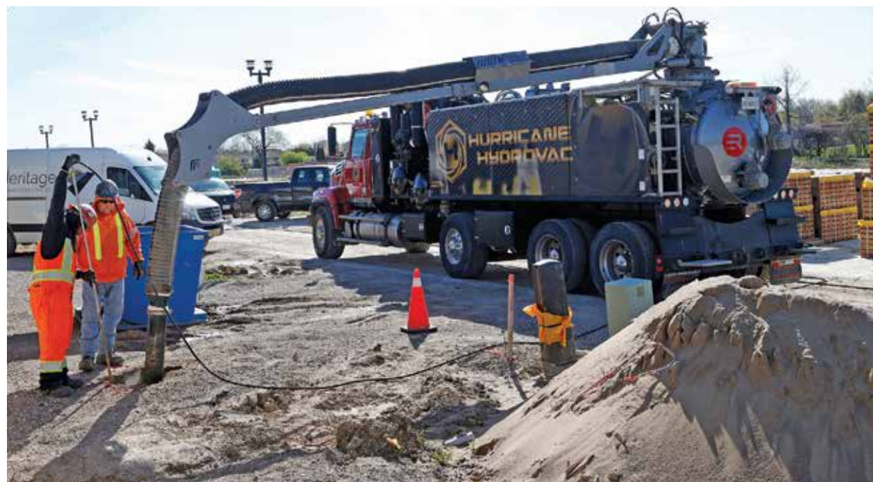
Carmon Geffs (left) and Tom Ross use the Rival hydrovac’s digging wand and boom to loose up dirt at a new home construction subdivision in Windsor, Ontario. Hurricane Hydrovac was on site to clear and make a trench so others could try and find where lines were cut by someone else so it could be repaired.
