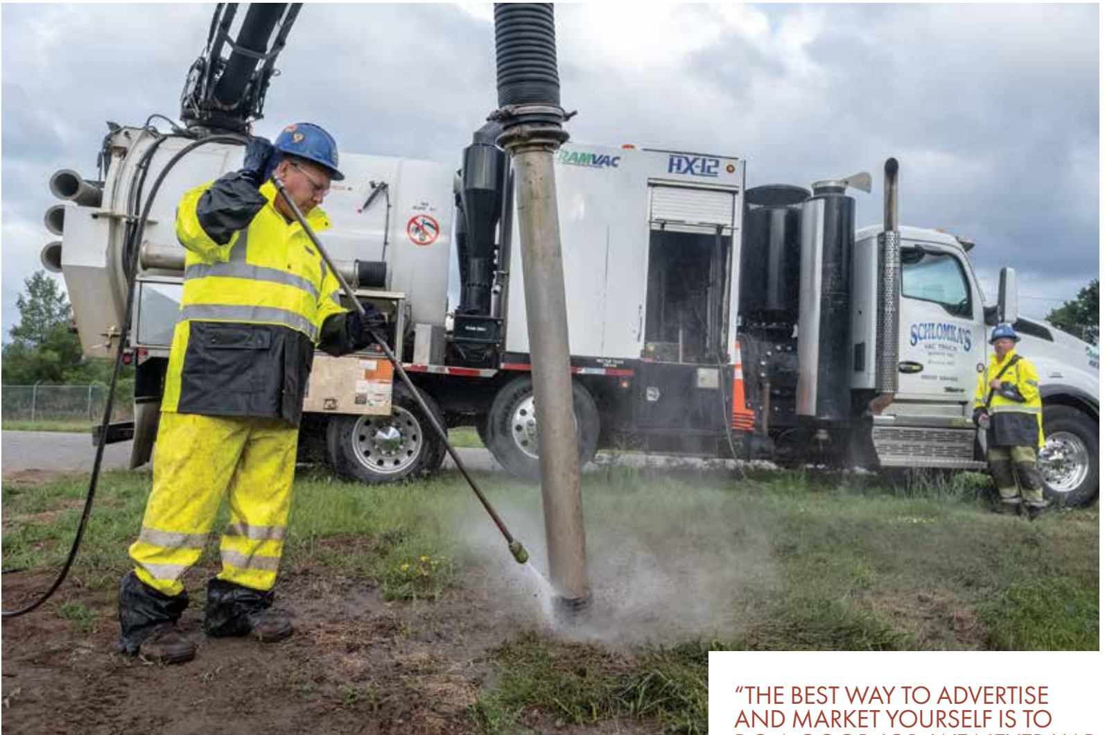
Operator Steve Taube demonstrates how they dig a hold using one of Schlomka Vac Truck Service's RAMVAC HX-12 vacuum excavators.
