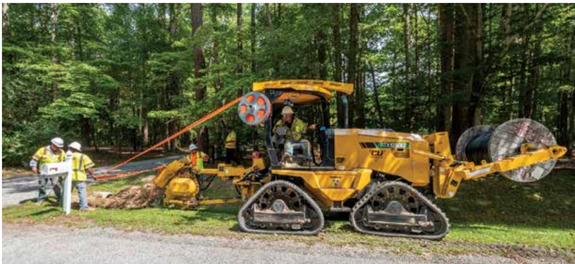
Complete Underground's full range of services covers the needs of commercial clients, municipal utility departments, and even residential properties.
