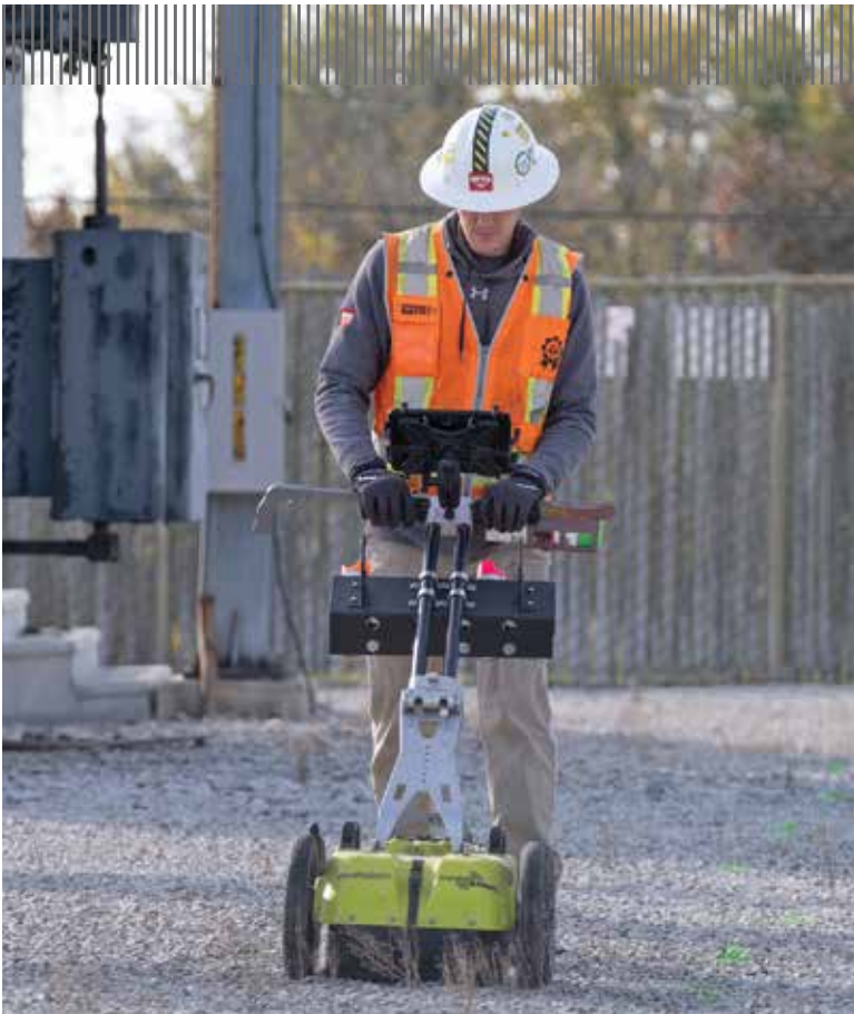
Schings uses an ImpulseRadar PinPointR to locate underground utilities at a substation. Crews from GPRS typically work solo unless a larger project requires more than one project manager.
