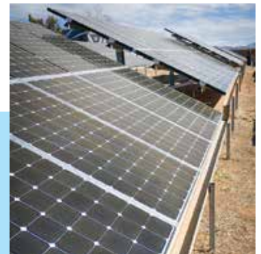
Solar array water catchment system located at Santa Fe Skies RV park.
