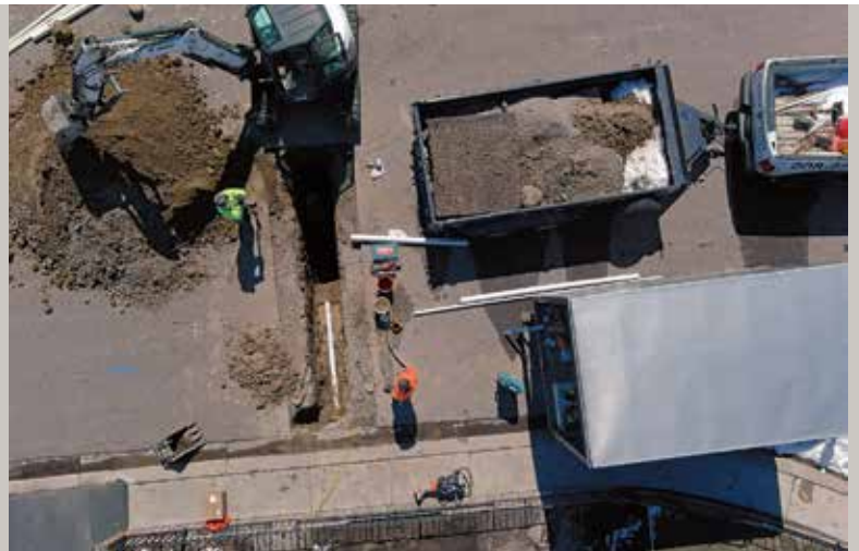
Drone view of a trench and pipe installation by Platinum Plumbing in southeast Idaho.
