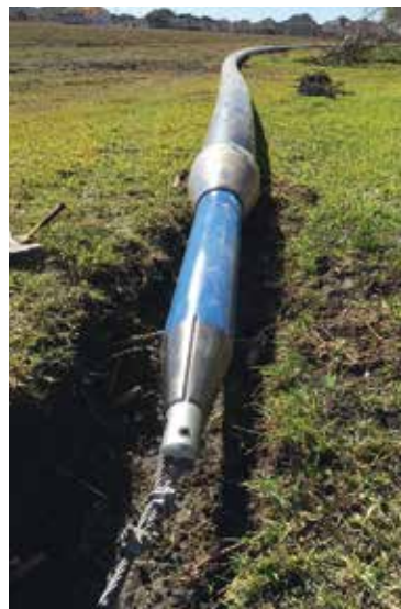
The pipe bursting approach enabled new HDPE pipe to be installed without damaging homeowners' properties.
