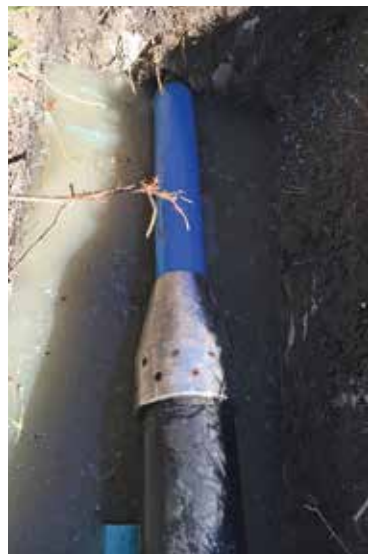
The pipe bursting process took place during a sewer system replacement project in a community southeast of Houston.
