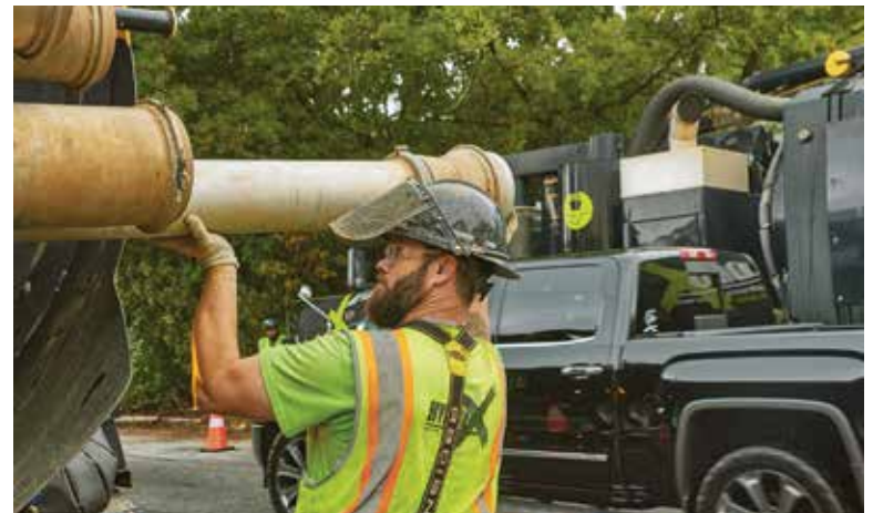
Neil Barrington removes a dig tube off the back of his truck for use on site.
