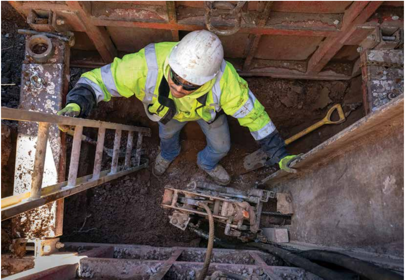
Scott Lamers Construction technician Rene Cortes uses a HammerHead PB30 to pull a cable that will be used to pull a new water and sewer line into a home. The company added pipe bursting to its service offerings 15 years ago and continues to see it grow.
