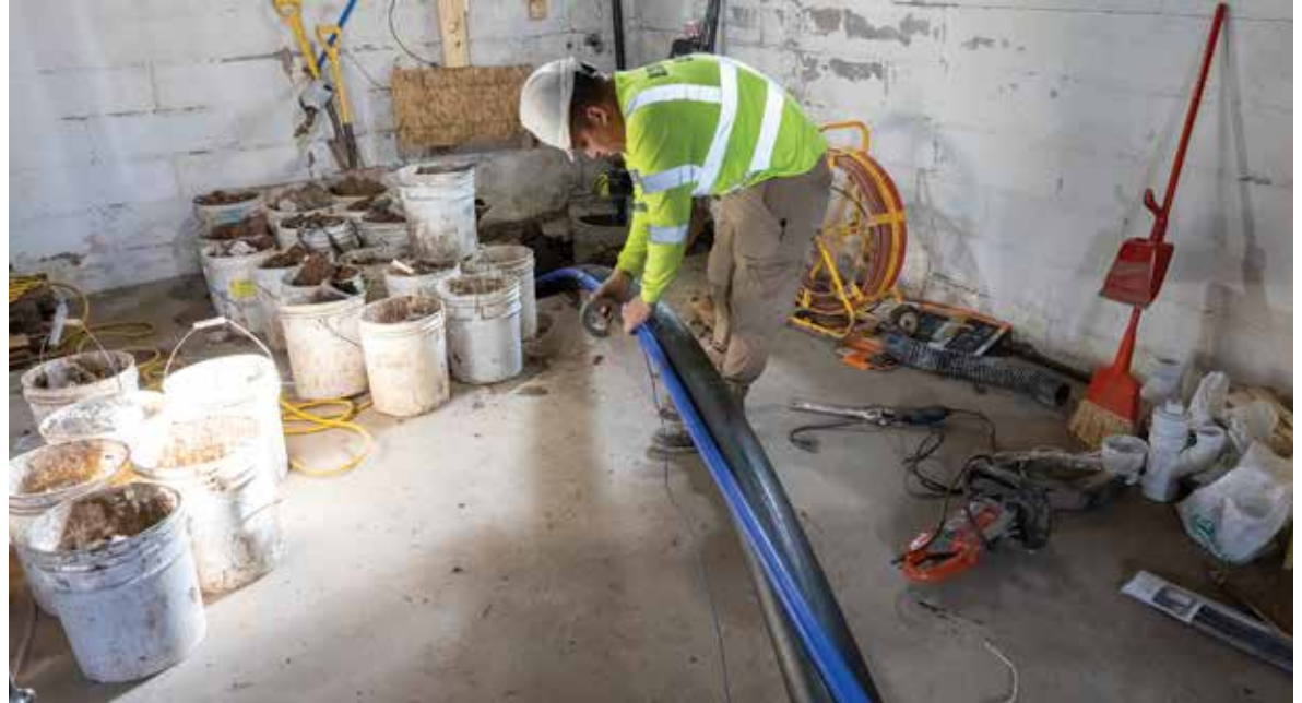
Technician Jose Leiva prepares a 4-inch HDP SDR17 sewer and 1 1/4-inch HDP SDR9 waterline that is being installed in a home remodeling project in Appleton, Wisconsin.
