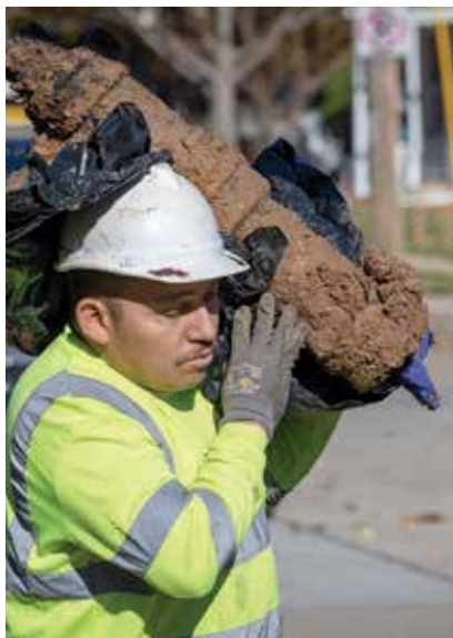
Leiva carries an old pipe segment from the job site. Crews were installing new lines in a residential property.
