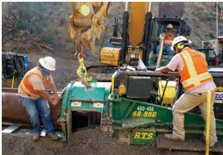
Craig Gunther (back) operates a Cat 336 excavator, providing leverage to a Barbco 48-950 auger-boring machine as Martinez (left) and Alan Rodriguez prepare it for operation.
