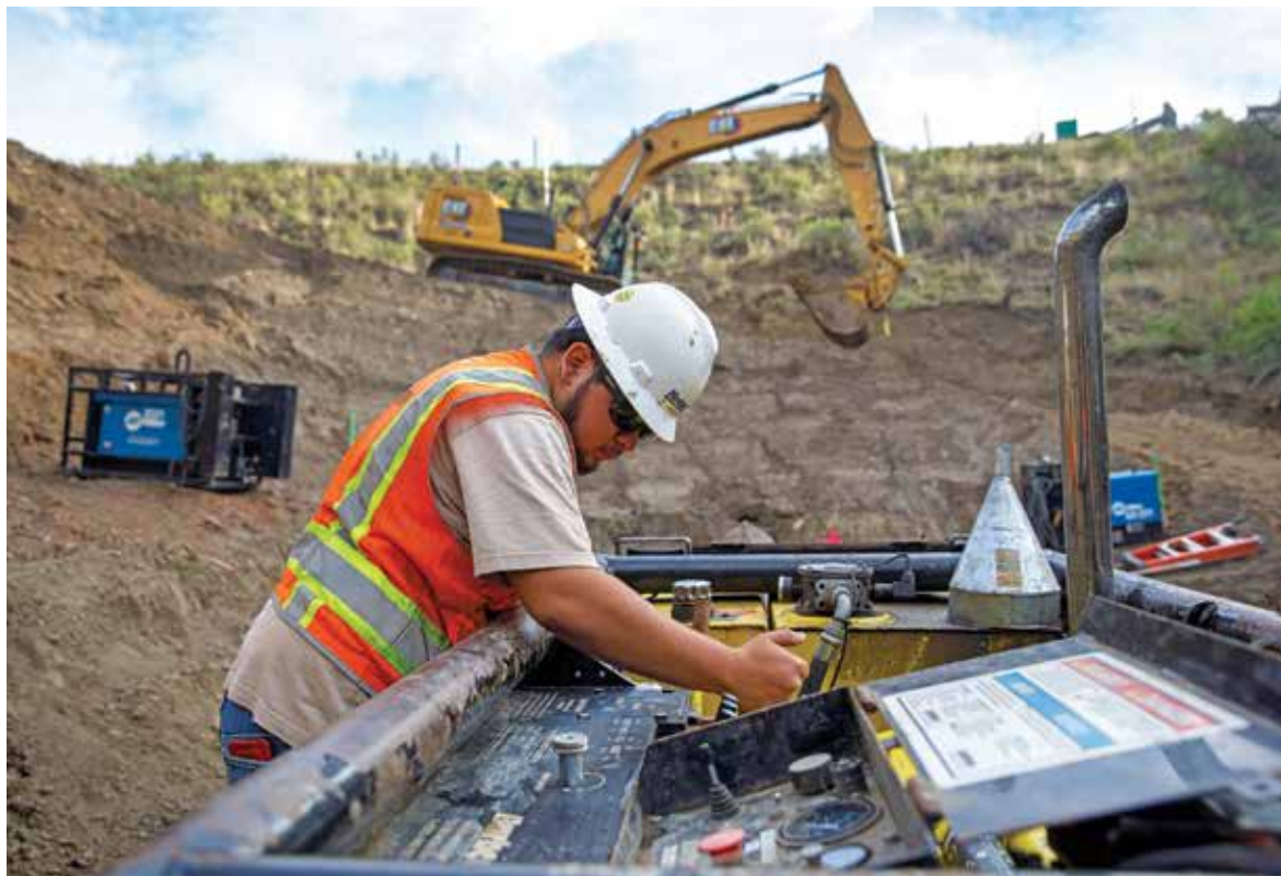
Juan Martinez at an auger-boring tunneling project in South Dakota. The company has also branched out into other trenchless technologies.
