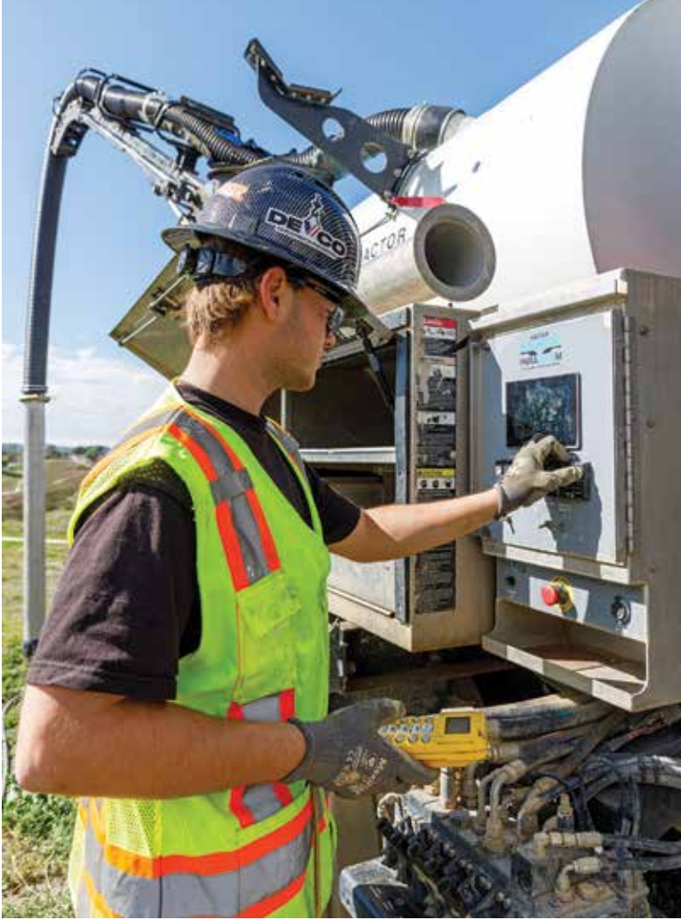
Drake Rossi sets up the HXX Paradigm (TRUVAC) hydroexcavator on a job site in Temecula, California. Hydroexcavation and HDD work are the mainstay of the company's business.
