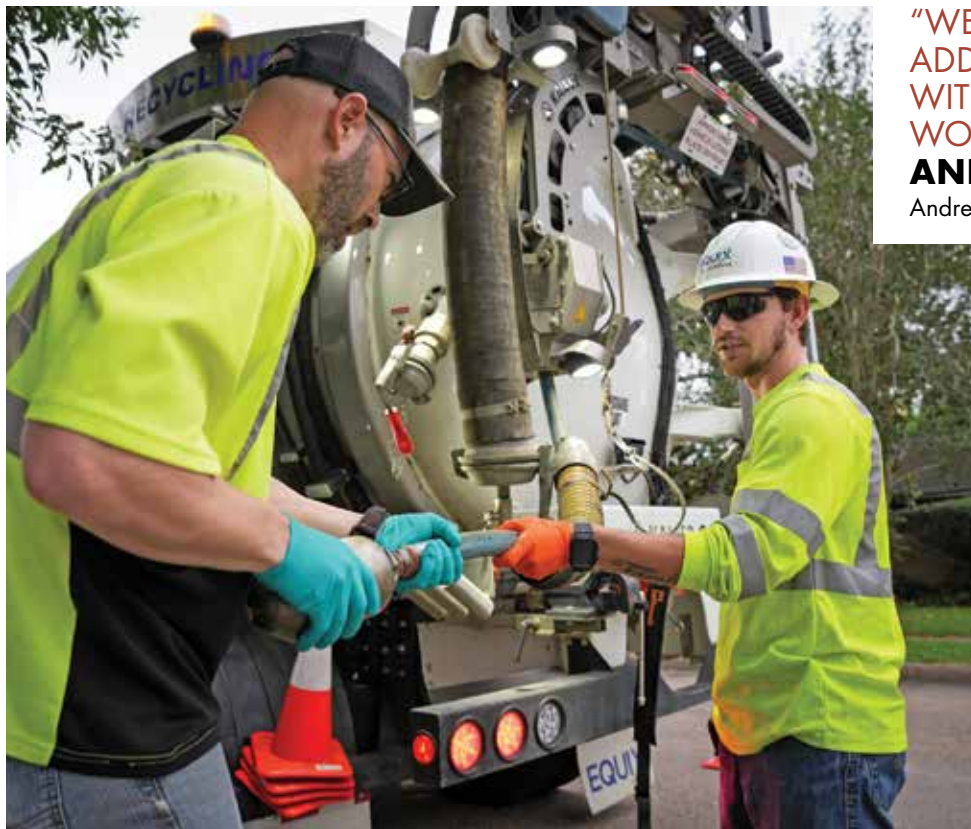
Ryan Albanese, left, an Equix Integrity crew leader, and Bryce Elliott, jet/vac operator, prepare to clear and inspect a sewer line using a 2023 KAISER AquaStar.
